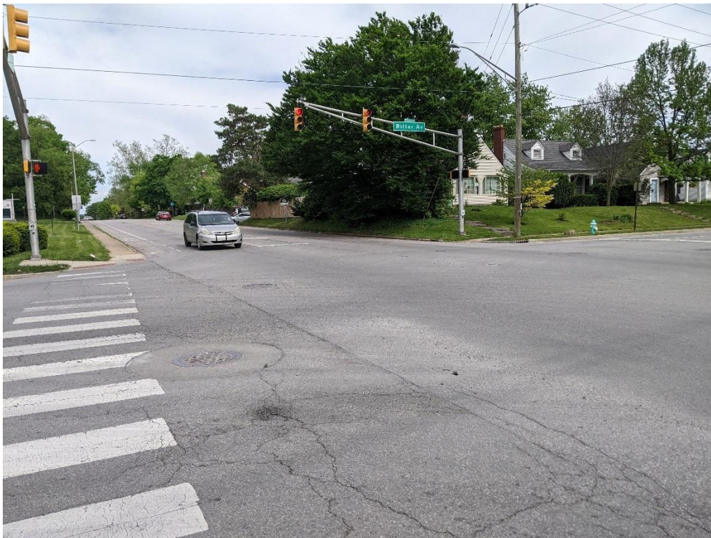
Figure 38. Photo of the northwest corner of 10 th and Ritter, looking east
